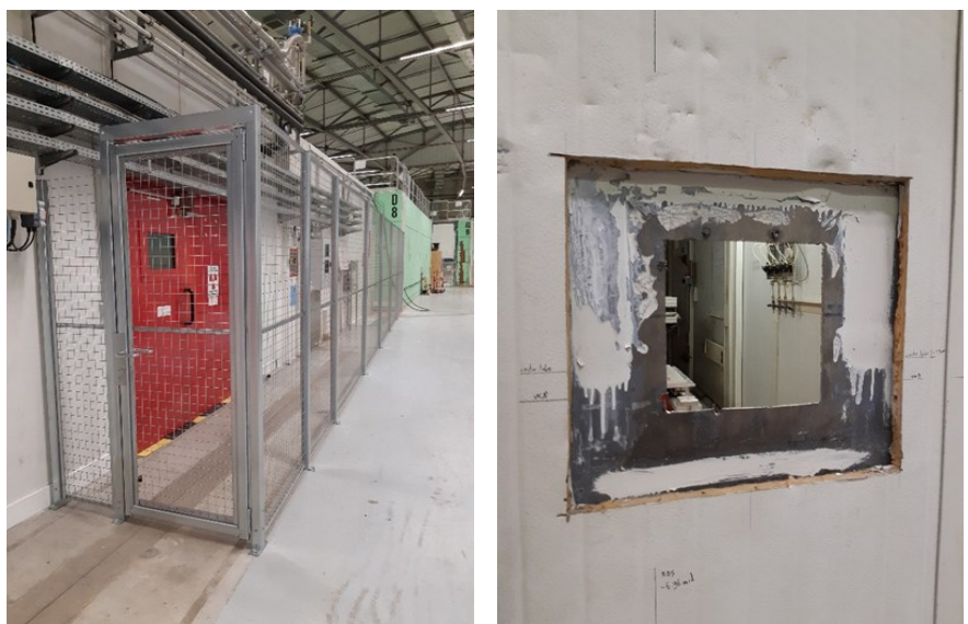
Figure 2: Left) The new fence contouring the Optic Hutch. Right) The lead shielding at the entrance of EH2 ready to be modified to allocate the transfer pipe in the new position.
